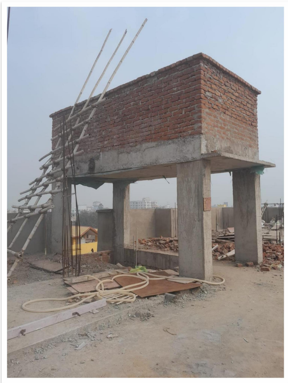
A BLOCK OVERHEAD TANK
